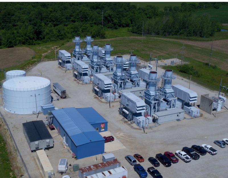
Greenville Generating Station
